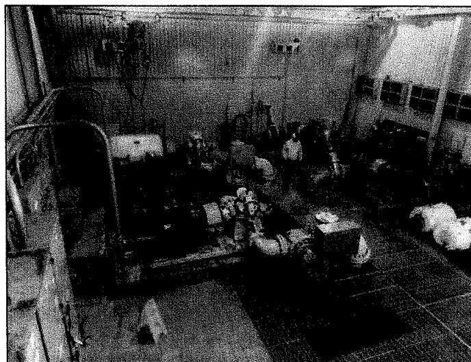
Photograph 1 (Elevated pump room floor-Eddy's Lane Pump Station)
